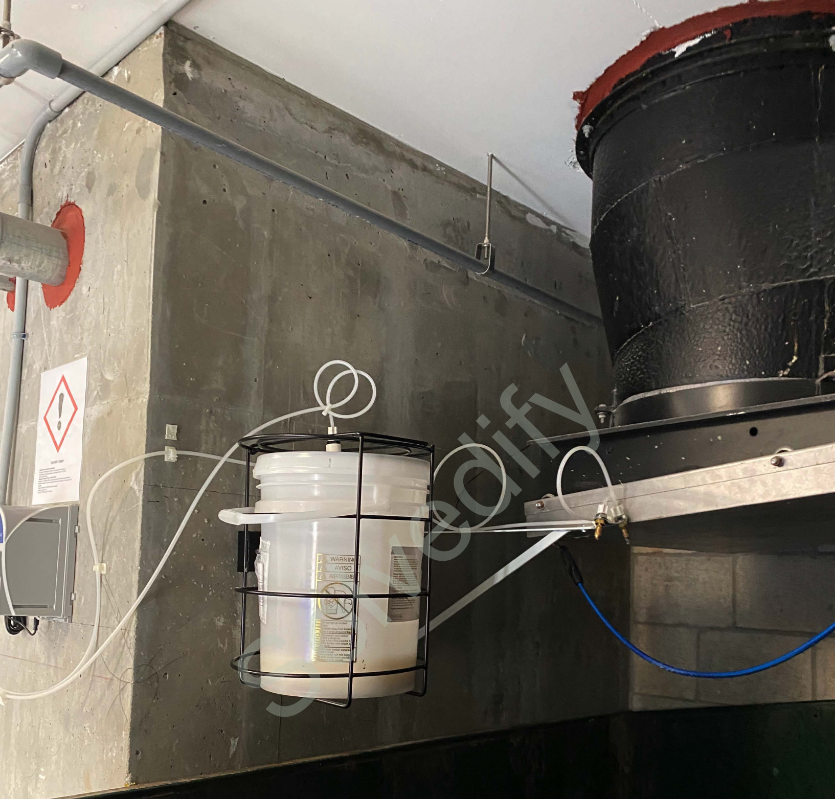
Installed at 1111 Central Naples, Fl. Luxury Apartments Vesta Property Management A/C closed garbage room
